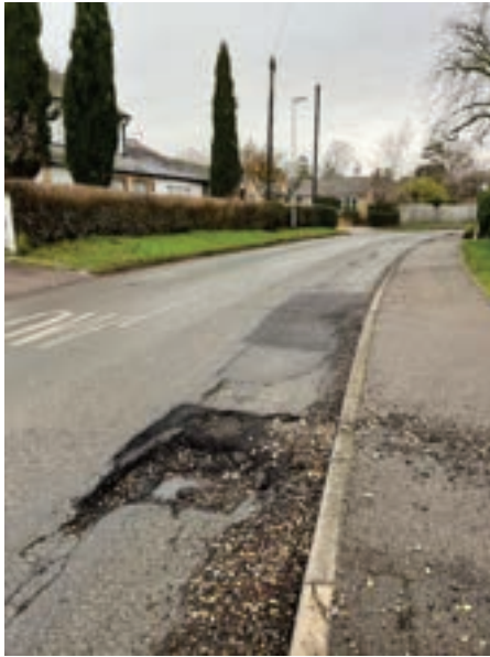
Image 6: Poor road conditions along National Cycle Route 11, Church Street, Stapleford
