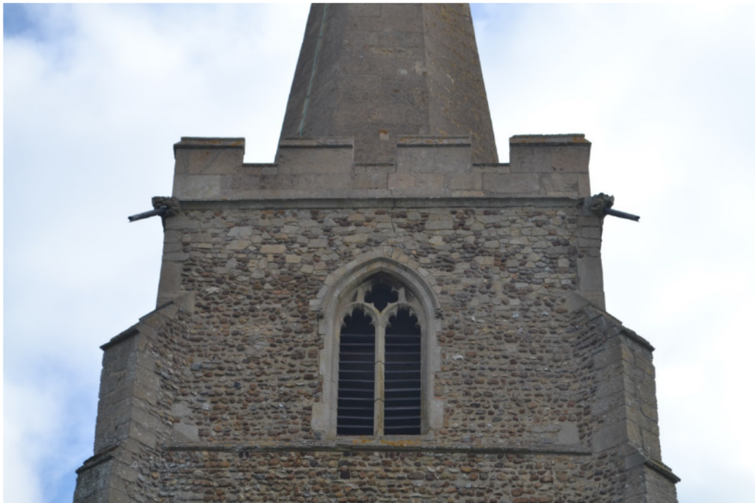
Photograph 6.7: All Saints Church. Cracks above the church window are visible in this photograph
