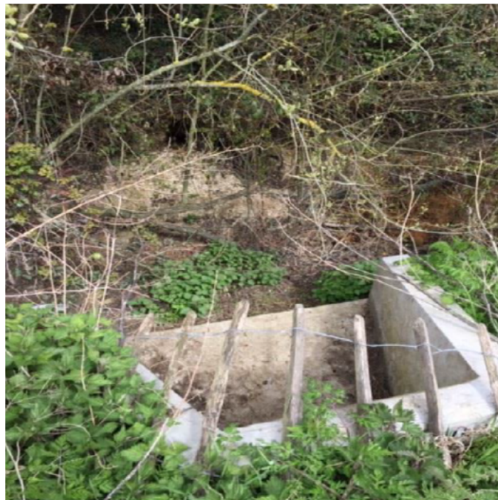
Photograph B.8: The Kingfisher Pond overflow pipe. April 2021
