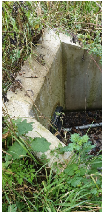
Photograph 5.11: Overflow pipe of the Kingfisher Pond, October 2020
